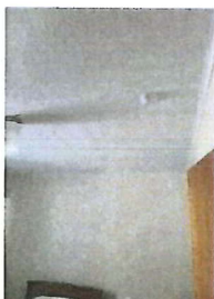
Smoke Alarm Photos
